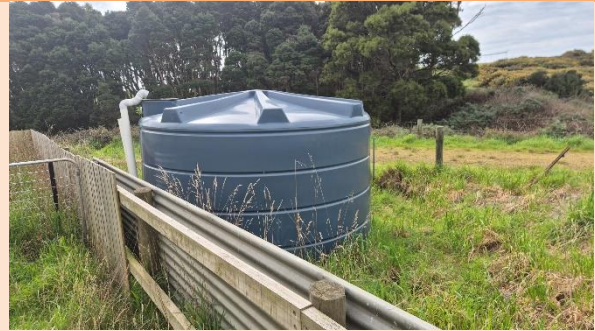
Existing tank – Lot 1 (non-compliant for fire fighting purposes)
